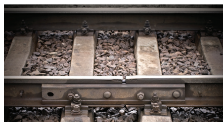
Figure 7.1 Gap in railway track
